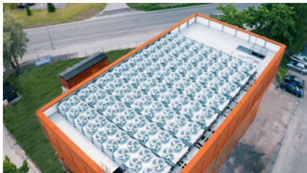
FIGURE 32. Energy collectors of Calefa heat pump system in Runosmäki, Finland (Picture courtesy of Calefa Oy)
