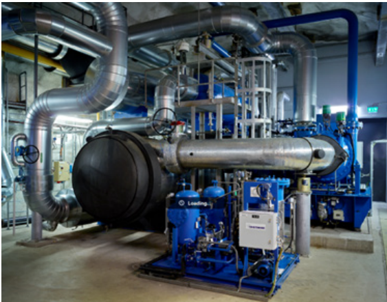
FIGURE 13. Friotherm heat pump in Katri Vala plant, Helsinki (Picture courtesy of Helen Oy)
