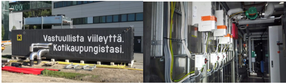
FIGURE 33. The transferrable CHC plant by Oilon (Oilon 2020 & Oilon 2022c)
