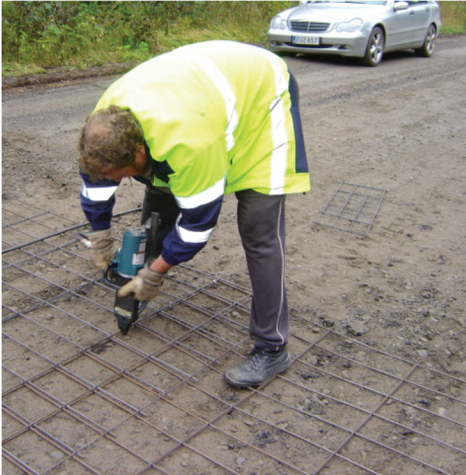
PICTURE 4. There is a patented method for installing the steel mesh, which has been developed further by the students of TUAS. Photo by Olli Heinilä.
