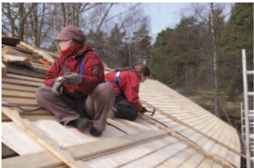
Maria Lumo and Enni Ellä nail shingles. Rows are kept straight with "riialauta" and comb board.
