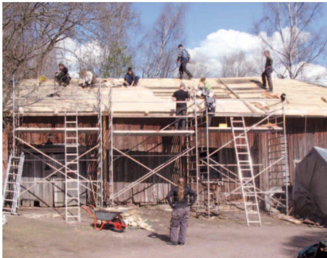
Students of restoration renew a shingle roof in Toijainen in 2010. Photos: Markku Hyvönen.
