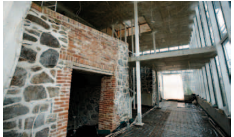
The former Viljandi manor barn, the current Estonian Traditional Music Center. Construction.
