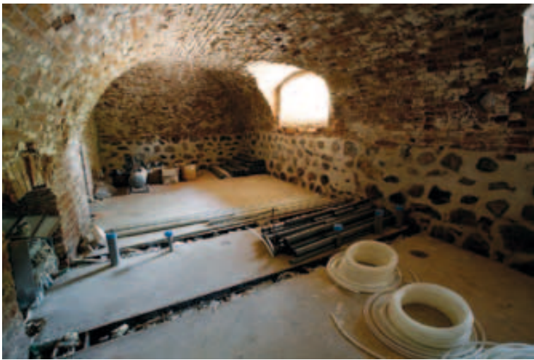
A fieldstone wall with lime mortar is easily the most common building material solution seen in the cellars and foundations of a century ago. The cellar space of the Pärimusmuusika Ait (Traditional Music Barn) in Viljandi in summer 2007. Photo: Urmas Volmer.
