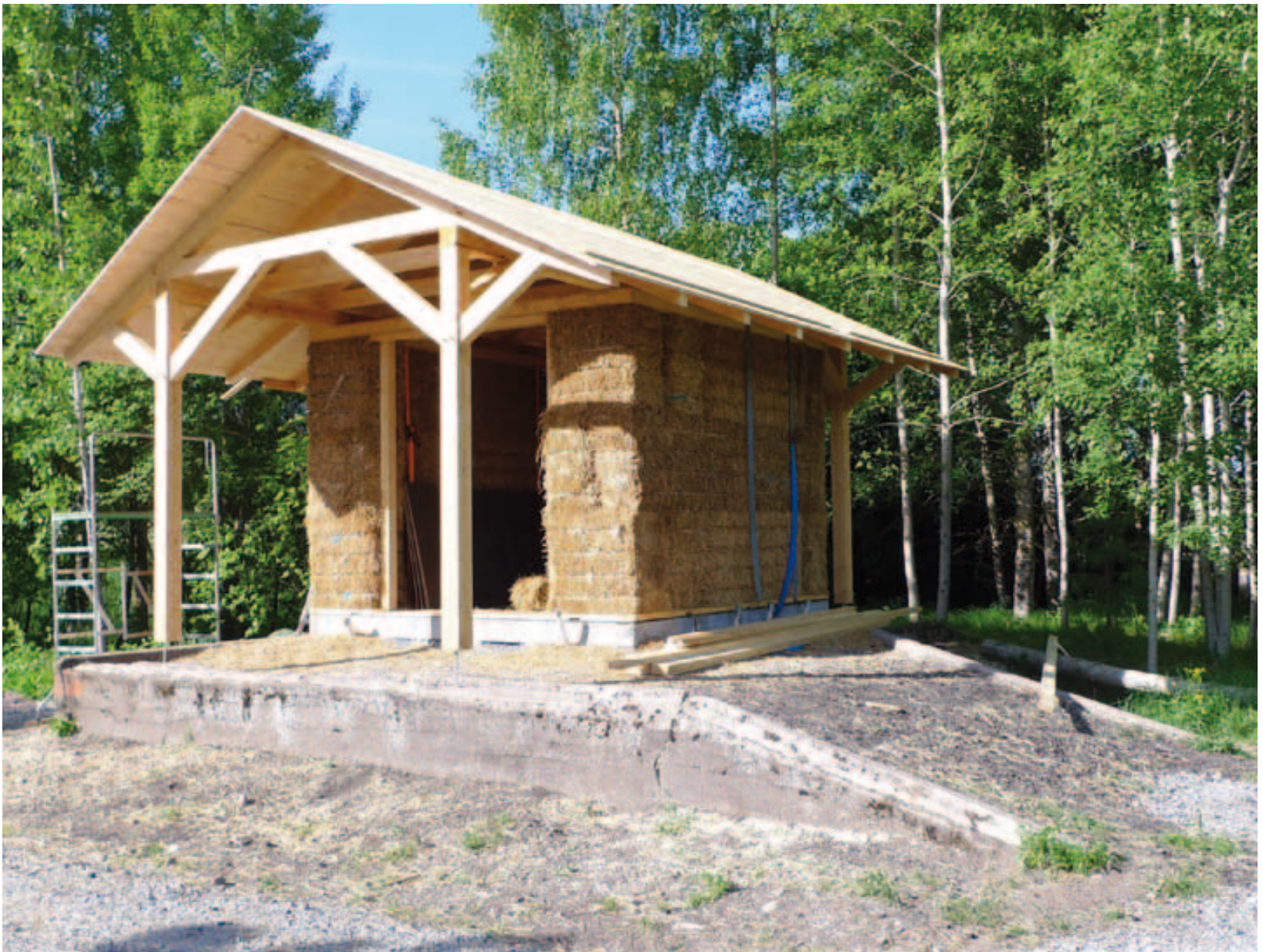
After bales are in place and compression is finished. Photo: Kasper Järnefelt.
