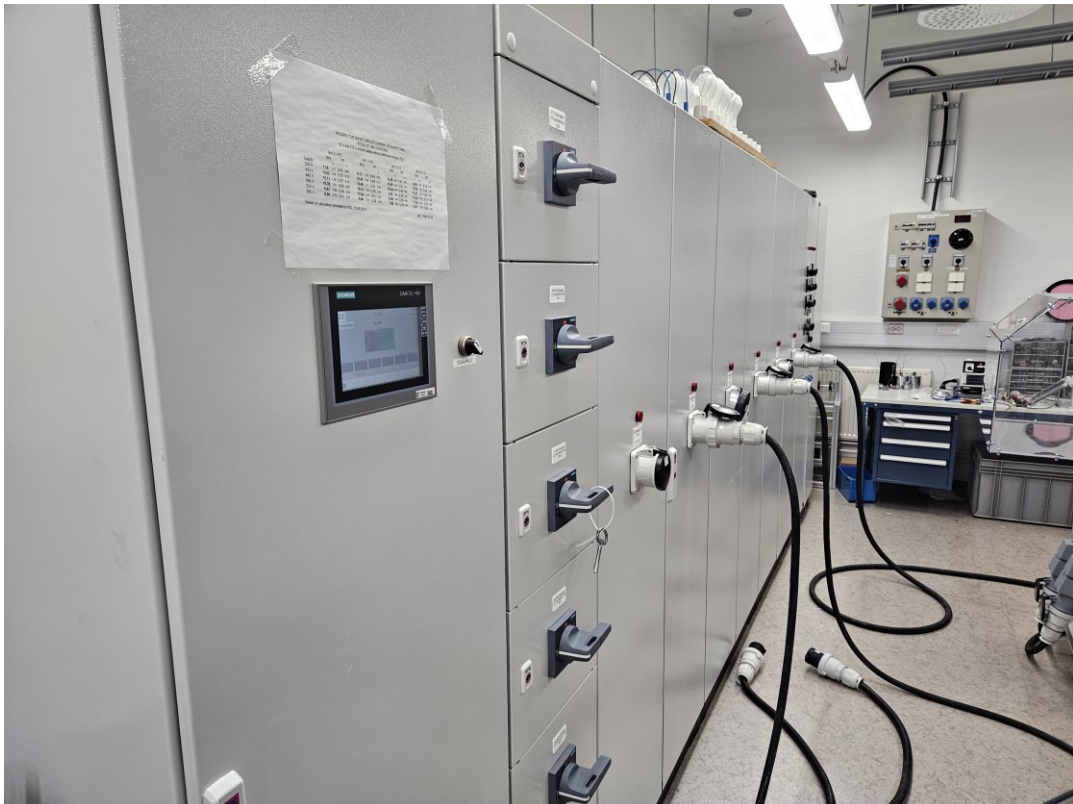
Figure 5. Testing room 227/228 125 A wall sockets and the control interface
