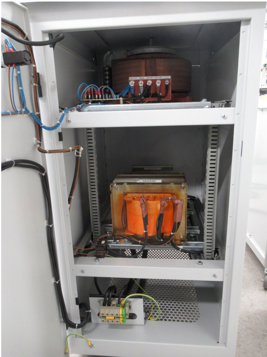
Figure 13. Voltage adjuster B maintenance panel open. Brush winding on top.
