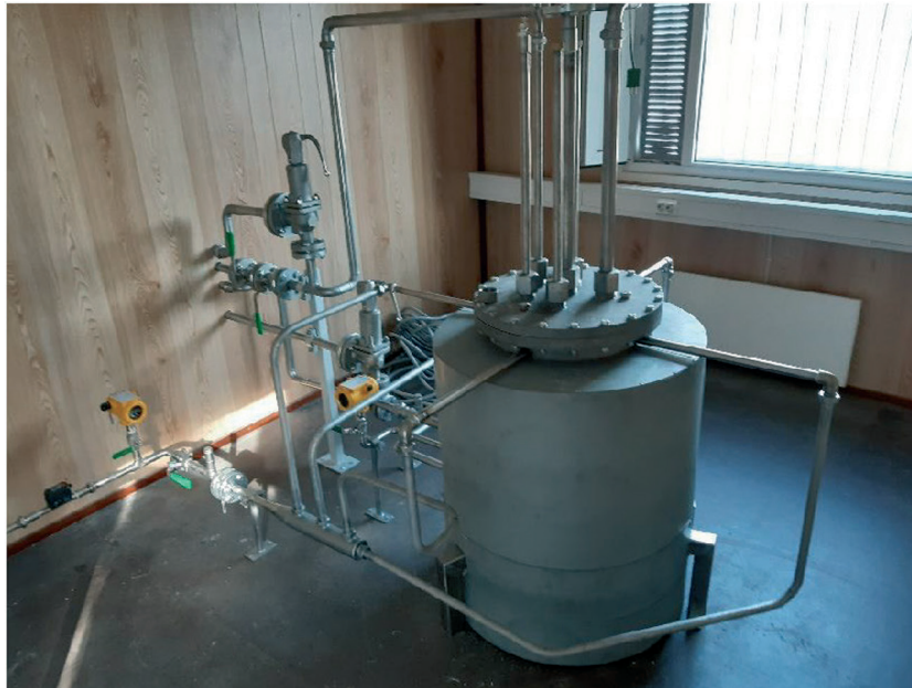
Figure 30. Savonia's thermochemical energy storage reactor (Image: Markku Huhtinen).
