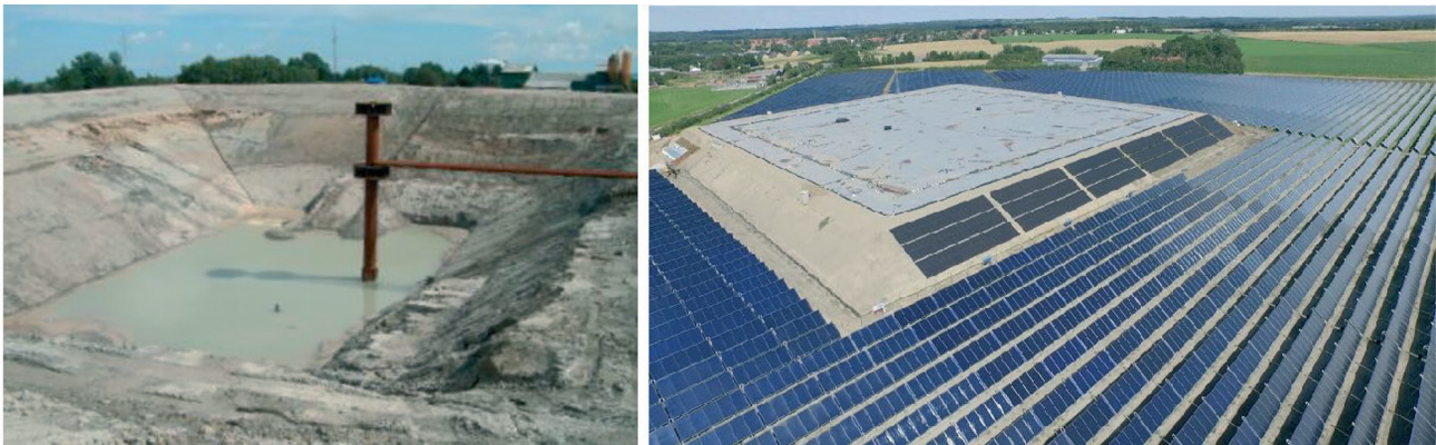
Figure 12. Left: Excavation of PTES at Marstal District Heating plant (Picture courtesy of Marstal Fjernvarme). Right: PTES at Gram District Heating plant (Picture courtesy of Gram Fjernvarme).
