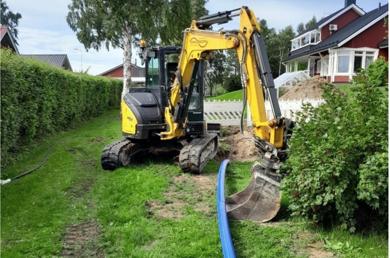
IMAGE 2. An example of a difficult pipe location inside private property lines [5].
