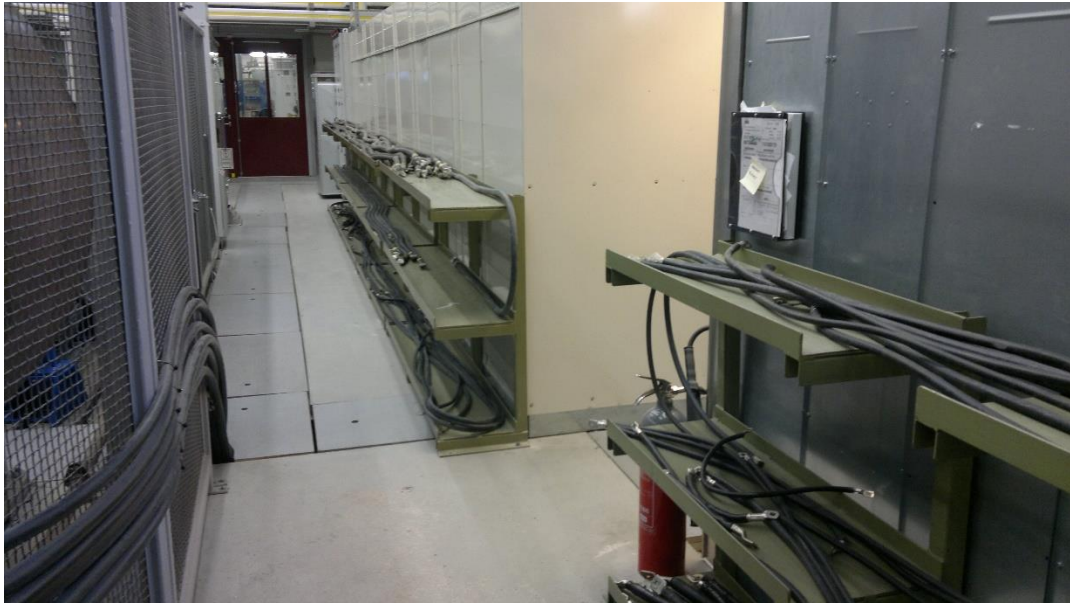
Picture 1. Large cables in the D-laboratory, ground plan number: 1
