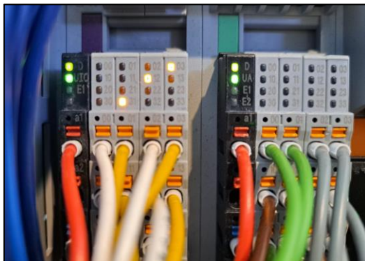
Figure 21: PLC output panel activation (Source: Author's own)
