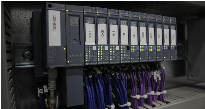
Figure 26- PLC and I/O modules in cabinet. (Source: www.logimatic.com )
