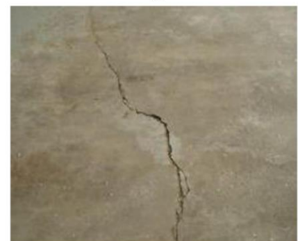
d. Concrete cracks
