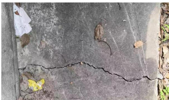
c. Pavement cracks
