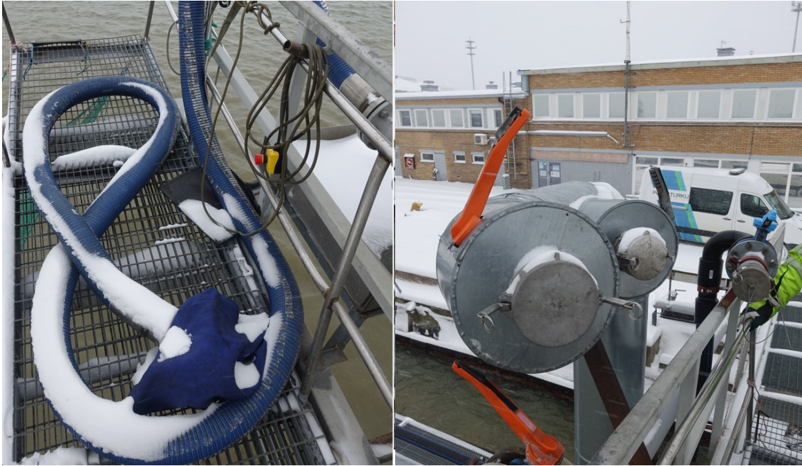
Picture 7 Pipelines used to supply water to cruise ferries on Port of Turku
