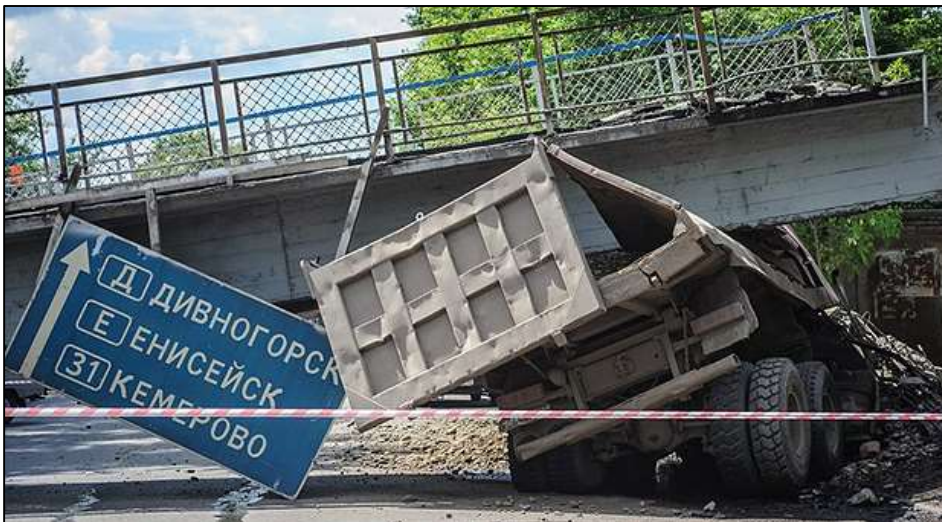
Image 12. the collapse of pedestrian bridge in Krasnoyarsk, Russia (Dela.ru 2014)
