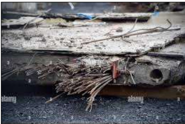
Image 17. The deck of Troja footbridge after collapse (Image: Vit Simanek)
