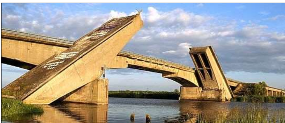
Image 21. Collapsed Palmburger bridge in Kaliningrad (Image: Rybakov Andrey)
