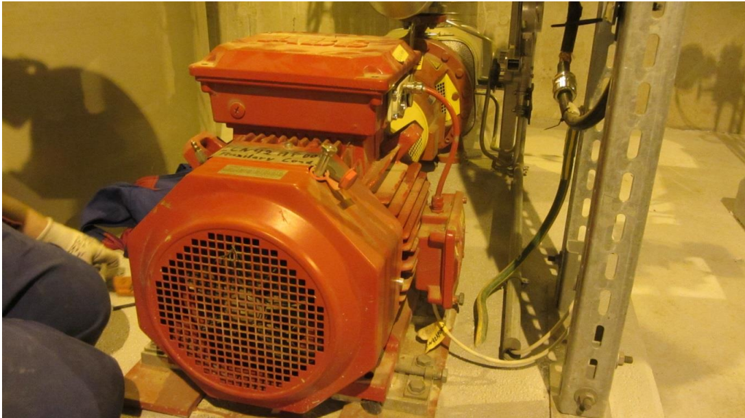
Figure 27. Some of the motors were only grounded through the incoming supply cable at the cable terminal box, like the 1LCN41AP001 (Cond Pp 1 AuxCondSys) motor in the picture. An additional grounding cable was connected to the case.
