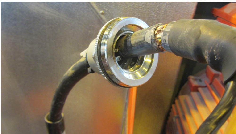
Figure 28. An EMC cable gland is used for connecting the supply cable to the cable terminal box. Many of the connection pins to the cable screen were broken at the 1HTC20AN001 (Bag filter preheating fan) motor. This gland was replaced.
