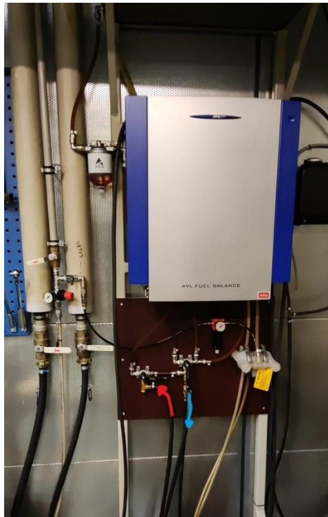
Figure 20. Picture of the fuel consumption device and the inlet (blue) and outlet (red) fuel pipes of the system (Author's own).
