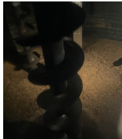
Figure 9. Metal coil in bioreactor at Stormossen Oy.
