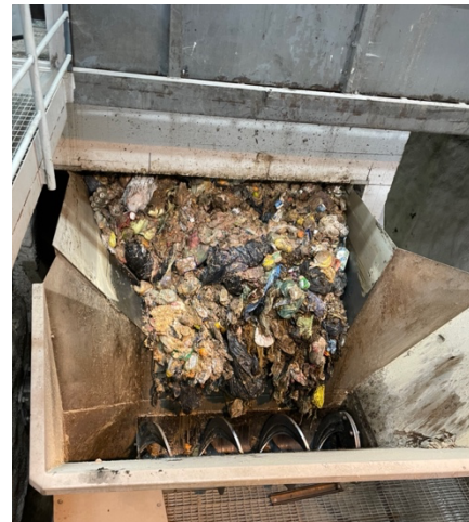
Figure 5. Screwtransporters feeding biowaste to crusher at Stormossen Oy.
