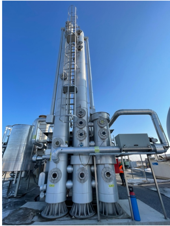
Figure 11. Gas upgrading unit at Stormossen Oy.
