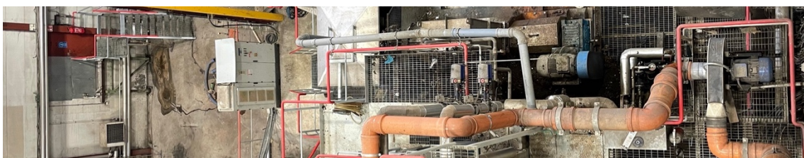
Figure 6. Ventilation pipelines at Stormossen Oy.
