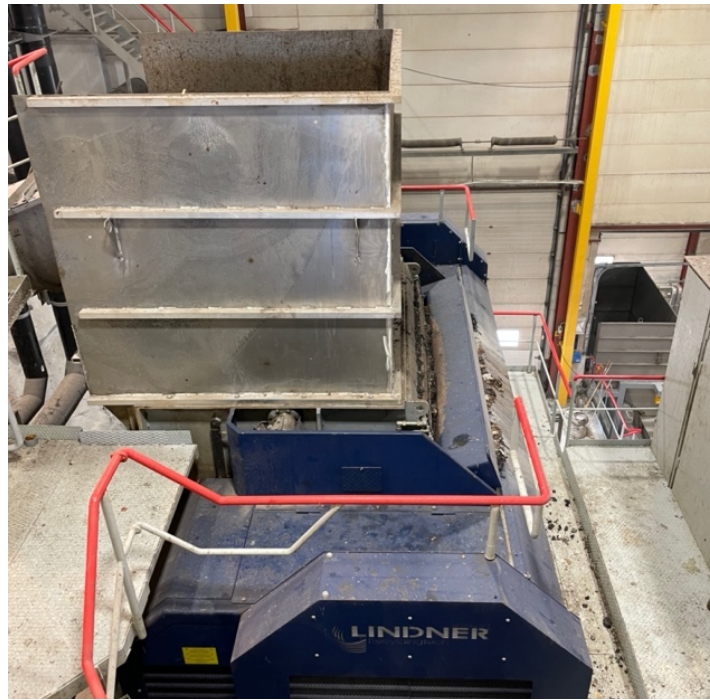
Figure 7. Biowaste crushing process at Stormossen Oy.
