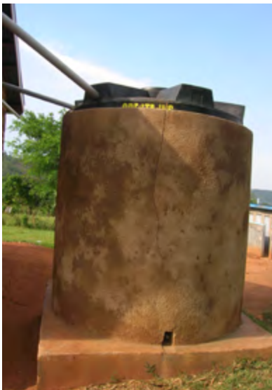
Picture 4. Water Tank Kibuuka Schools, Mpigi, Uganda (photo: Merja Seppälä 2008).
