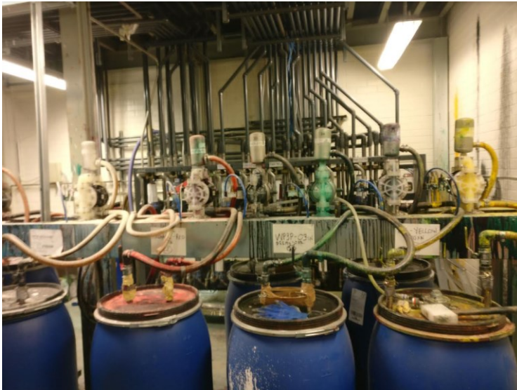
Figure 8. Stations on the first floor with the pumps seen in the background.
