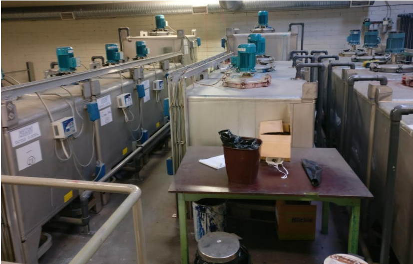
Figure 9. Stations on the second floor of solid containers of 1000 and 1500 liters
