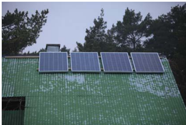
Figure 17 PV array mounted on cottage's roof
