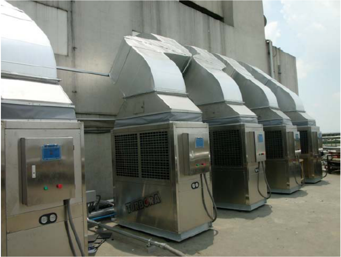
Figure 12: Heat Pump on the roof top
