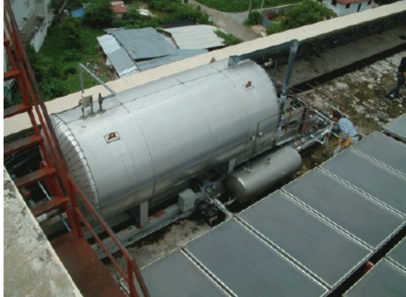
Figure 7: Storage Tanks in a Closed-Loop Force Circulation System
