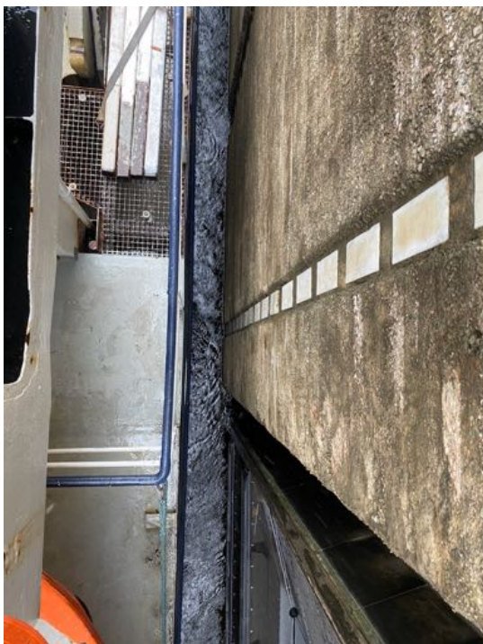
Figure 1: Horizontal lock clearance of a Saimax vessel. Picture from starboard side where port side is leaning against the lock wall. (Antti Tasala, 2021)
