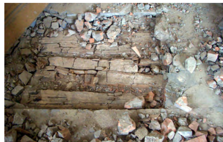
Figure 3.2. Seidla Manor. Floor boards are cracked by fungi. The topmost layer of bricks and plaster has not allowed rising damp to evaporate from the underlying wooden construction.
