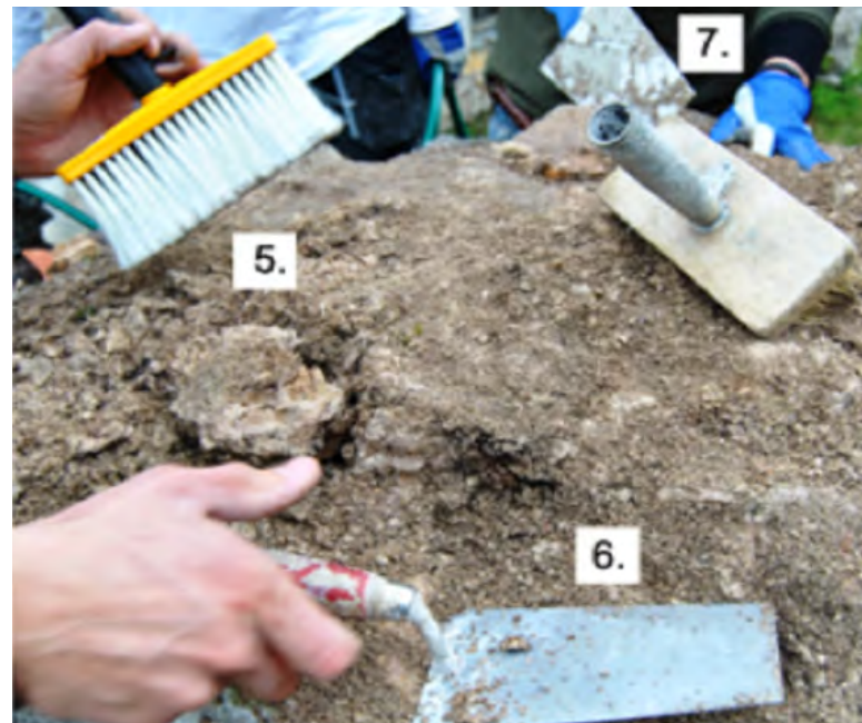
Figure 2.11. More tools: brushes (5)—used to wipe off sand and also to even out mortar on the sides of the posts; trowels (6)—used to apply the mortar onto the wall; waterproof gloves (7)—used when handling the mortar to prevent direct contact with lime; tape measures used for documentation.
