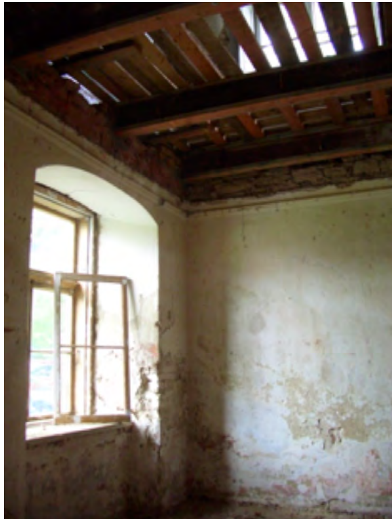
Figure 3.39. In some of the rooms at Seidla Manor there was neither ceiling nor cornice. Everything needs to be rebuilt.
