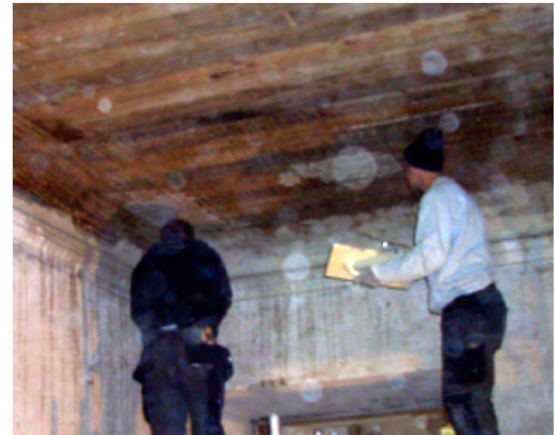
Figure 3.46. We were given a chance to try the traditional method of plastering the reconstructed cornice. This job is definitely something for experts!
