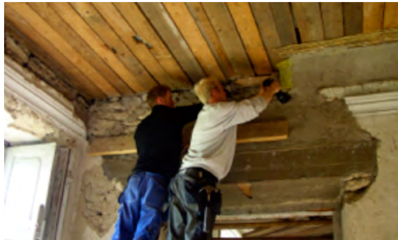
Figure 3.44. Reconstructing a cornice in one of the badly damaged rooms on the upper level.
