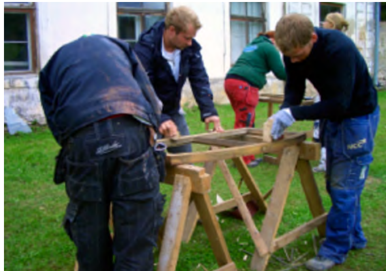
Figure 3.35. Sandpapering was quite easy as there was only one coat of paint to be removed and the wood was mostly in good condition.
