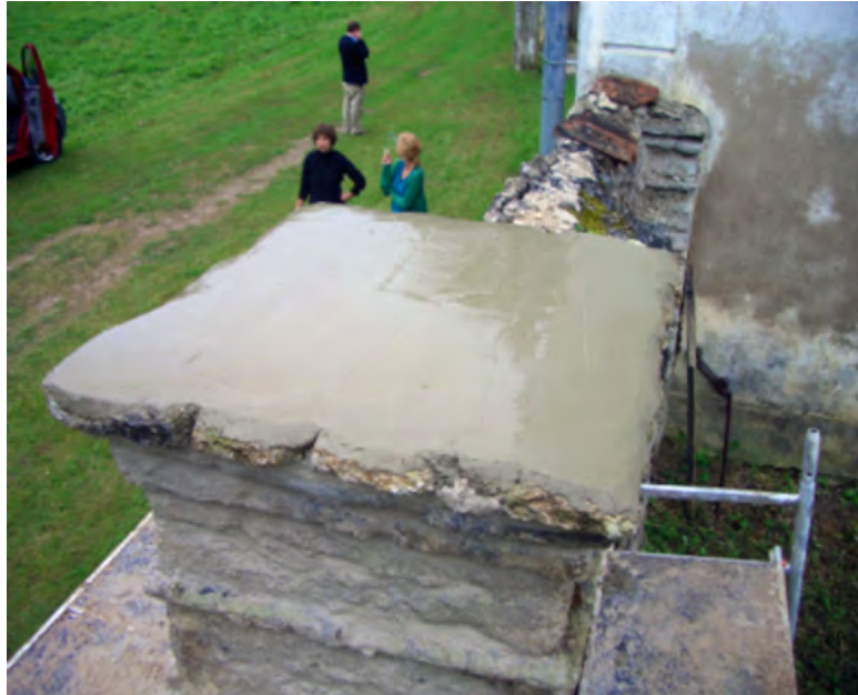
Figure 2.15. The broken flagstones on top of garden posts A and B had to be replaced with a topping of cement mortar because similar new stones were not available.
