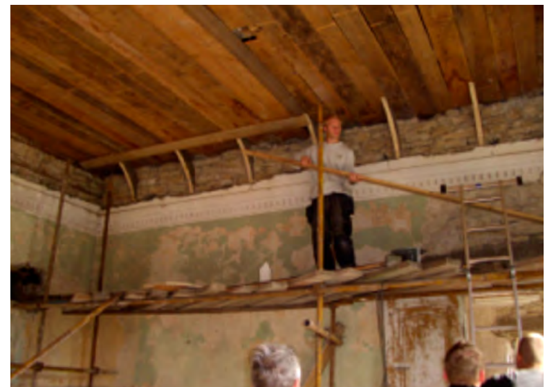
Figure 3.43. In the upper hall: new consoles are in place and planks are being attached to these. We finished the woodwork for the cornice along one wall.
