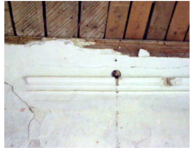
Figure 3.40. Plaster is removed from the ceiling and partially from the cornice. The ceiling needs insulation and the attic floor is missing, too. However, the timber frame of the cornice is most likely in good condition. The shape of the old cornice is possible to replicate.
