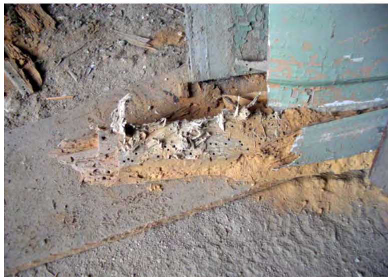
Figure 3.3. Seidla Manor. Top left: brown rot; center: white rot and destruction by wood boring insects.
