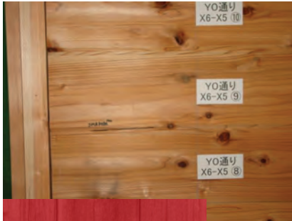
FIG. 1.20 A CRACK NEAR A OPENING
