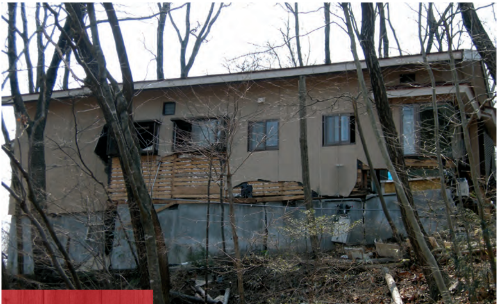
Pic. 1.10 A DAMAGED WALL OF A NEARBY HOUSE
