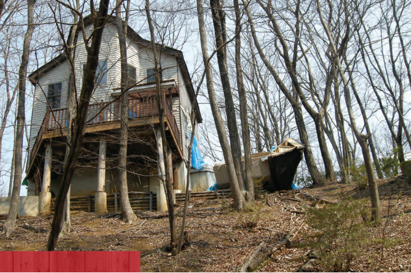
Pic. 1.11 A PART OF WALL FALLEN
