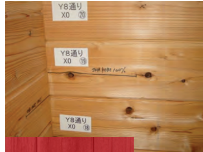
FIG. 1.21 A CRACK NEAR A NOTCH
