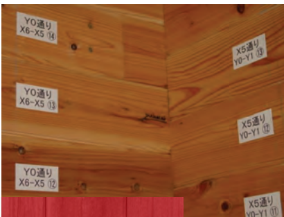
Pic. 1.18 A CRACK NEAR A NOTCH
