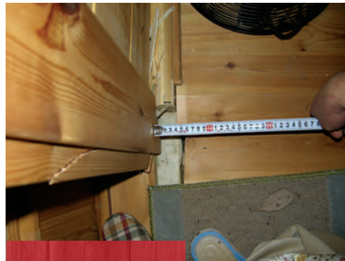
PIc. 1.7 ABOUT 60MM SLIPPAGE
