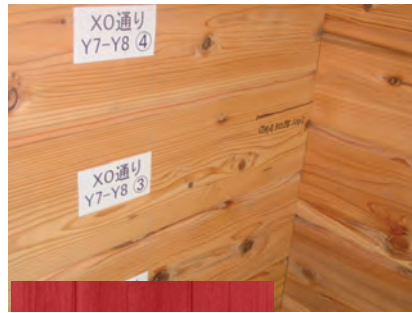
Pic. 1.17 A CRACK NEAR A NOTCH
