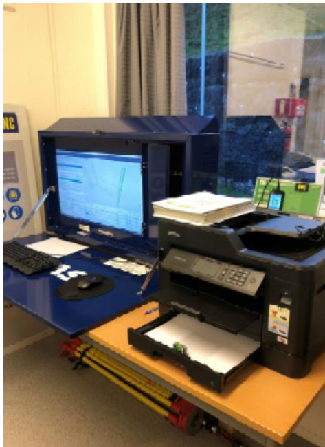
Figure 31: BIM- Station at the construction site (Copyrights for Sweco company with the permission of the author's use only).
