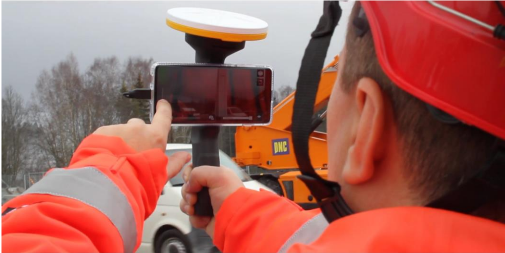
Figure 42: Site team member using SiteVision to visualize the column alignment on-site (Copyrights for Sweco company with the permission of the author's use only).
