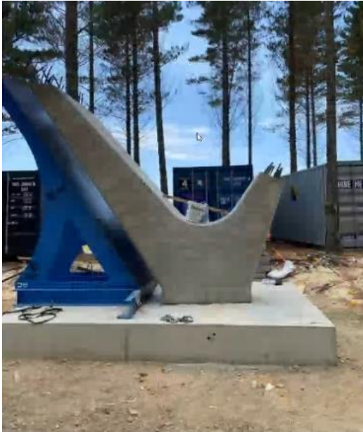
Figure 43: The complex corner foundation (precast concrete unit) in the construction site after casting (Copyrights for Sweco company with the permission of the author's use only).
