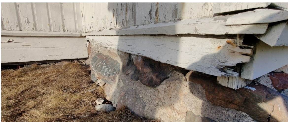
Figur 79 Brädet under dropplisten murket (Isaksson 2021)
