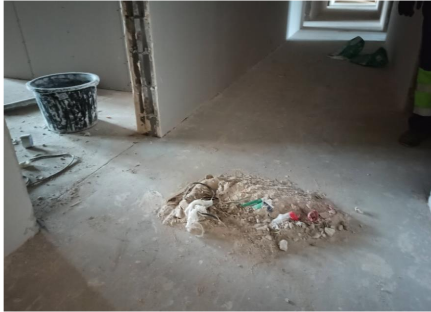
Figure 3.8 Unfinished cleaning of the workplace.
