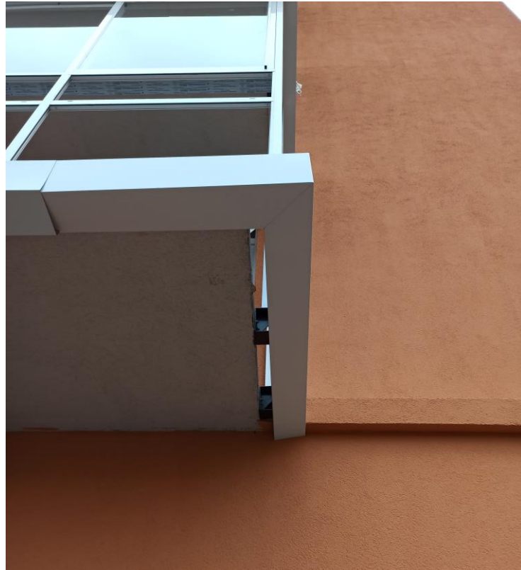
Figure 3.11 Steel profile solution to a balcony design mistake.
