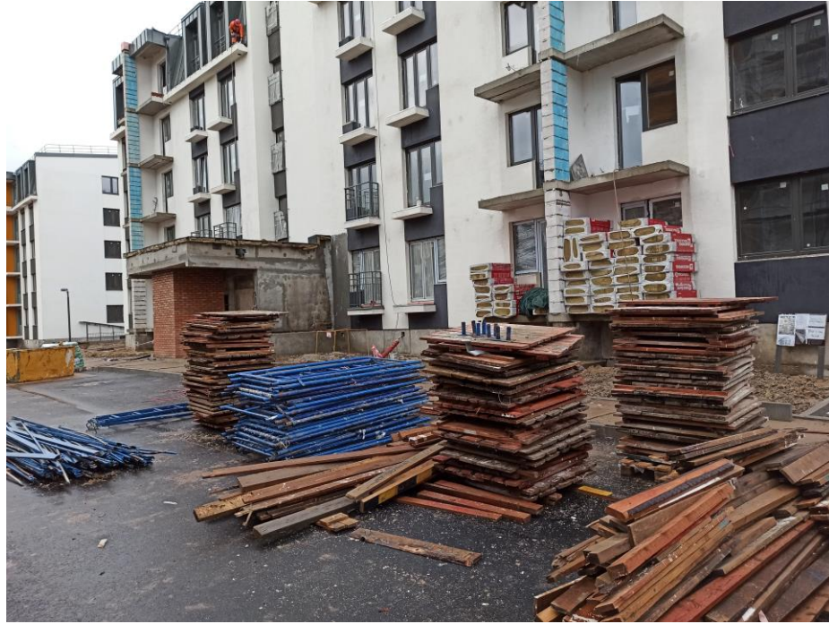
Figure 3.14 Reusable scaffolding and questionable insulation storage
