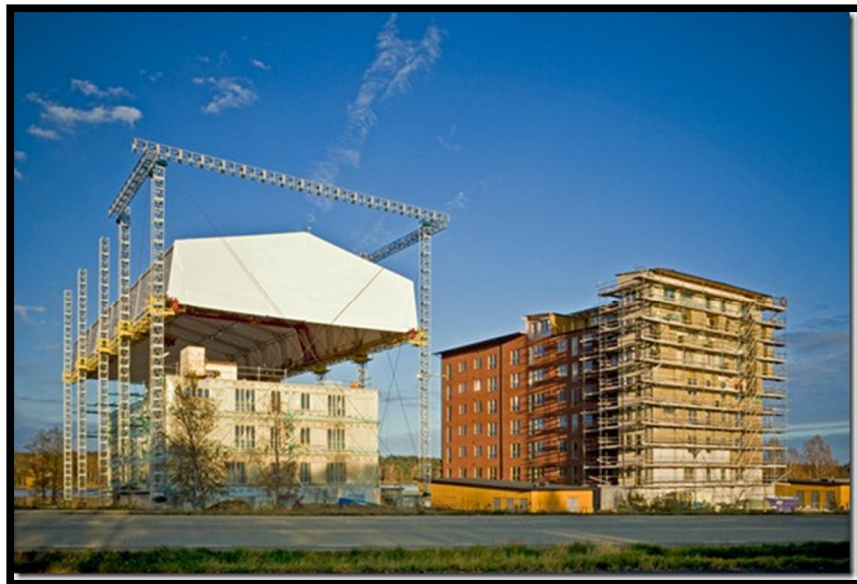
Figure 2.18 LIMNOLOGEN complex. Movable roof under the last building (SESAC, http://www.concerto-sesac.eu/spip.php?rubrique141 )
