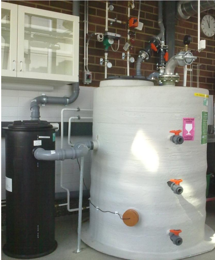
FIGURE 6. Biowaste preservation installation in the TAMK greenhouse (Photo: Luis González Martos 2011)
