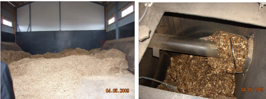
Figure 3.2. Woodchip stock and plenum chamber with feed screws in the boiler room. Photos: Martti Härkönen
