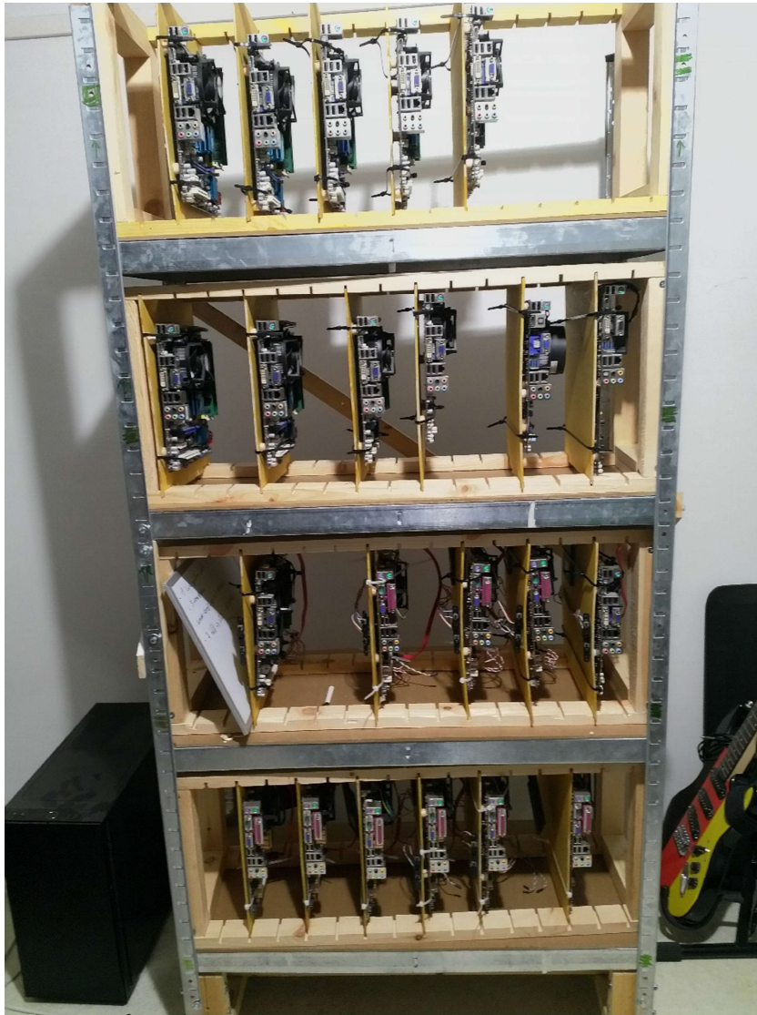
Figure 8. DIY server rack expanded
