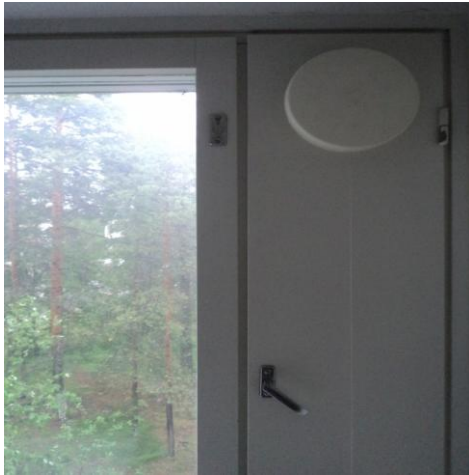
Figure 2. Inlet valves in windows .
