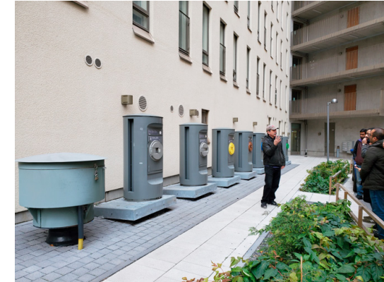
Figure 3 8-Waste Pipeline Rööri (Author)
