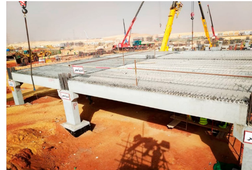
Figure 2.8 First Precast Garage in Egypt - New Capital Opera 500 Project (By the Author)
