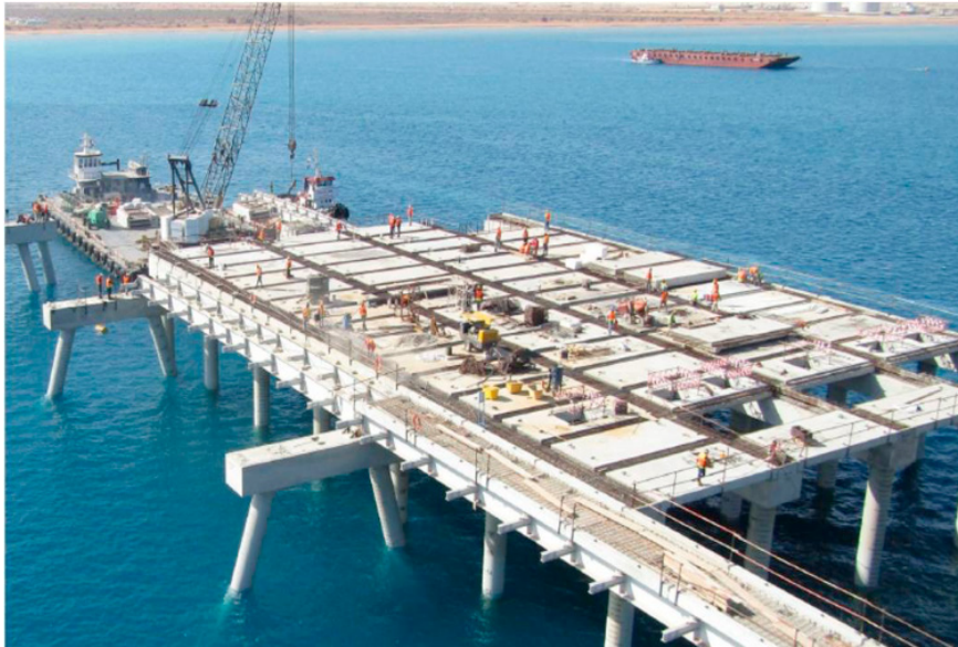
Figure 2.9 Production of precast Element for a product hub in Ain Sokhna city- ASPH (By the Author)
