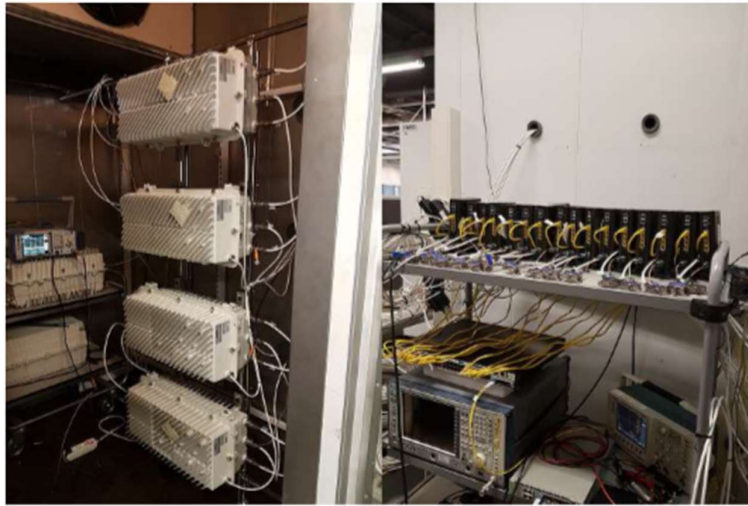
Figure 9 Picture of the environmental chamber on the left and the modems outside on the right
