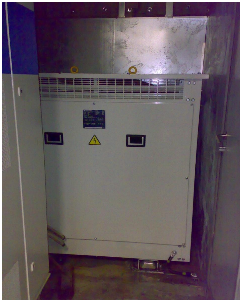
Figur 8. Transformator. (Eget arkiv, 2010b)
