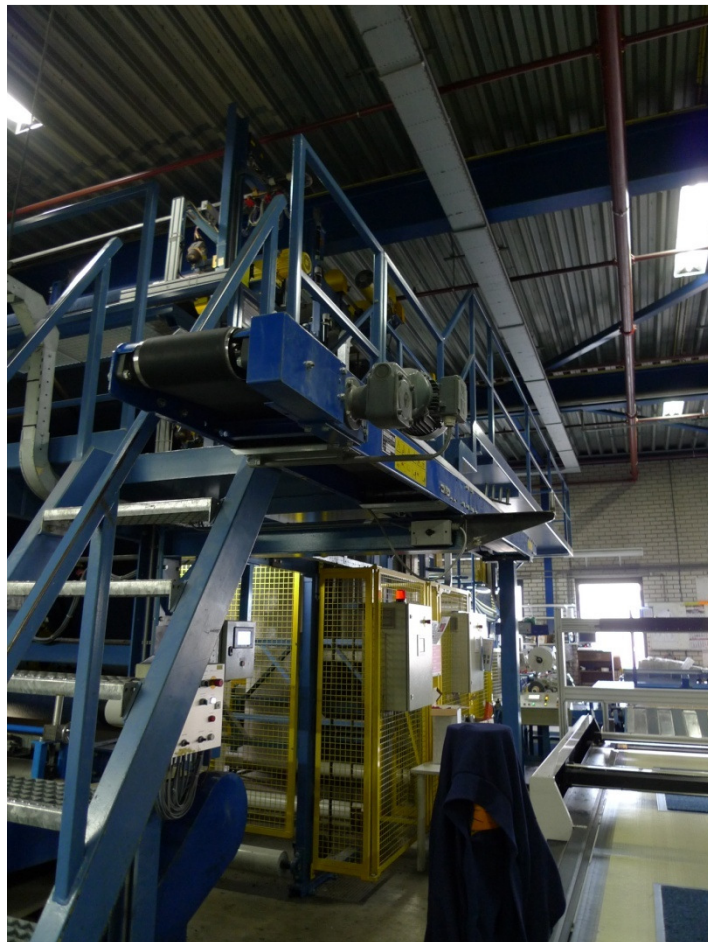
Figure 38: PVC waste conveyer
