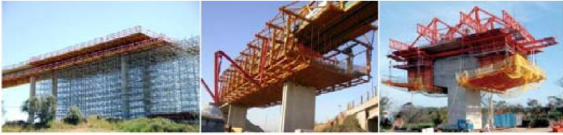
Figure 29: Traditional, incremental, and cantilever bridge construction methods. Source (P. Martins & Z. Sampaio, 2011)
