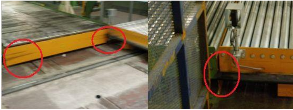
FIGURE 10. Too long rubber emergency stop plates, which are touching the conveyor
