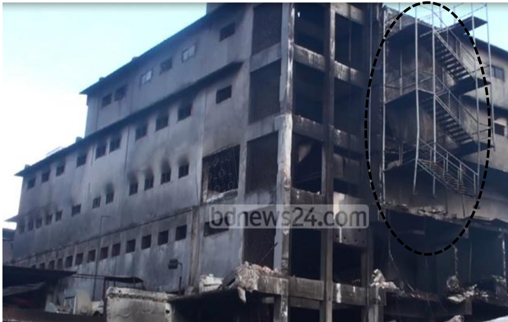
Figure 11: Tampaco Foils Ltd condition after fire hazard (bdnews24, 2016).
