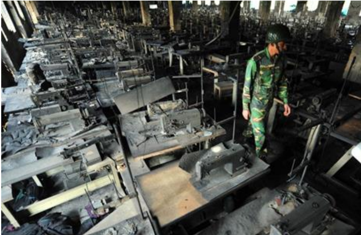
Figure 6: View of Tazreen Fashion Limited from inside after the fire hazard (Getty, 2012).
