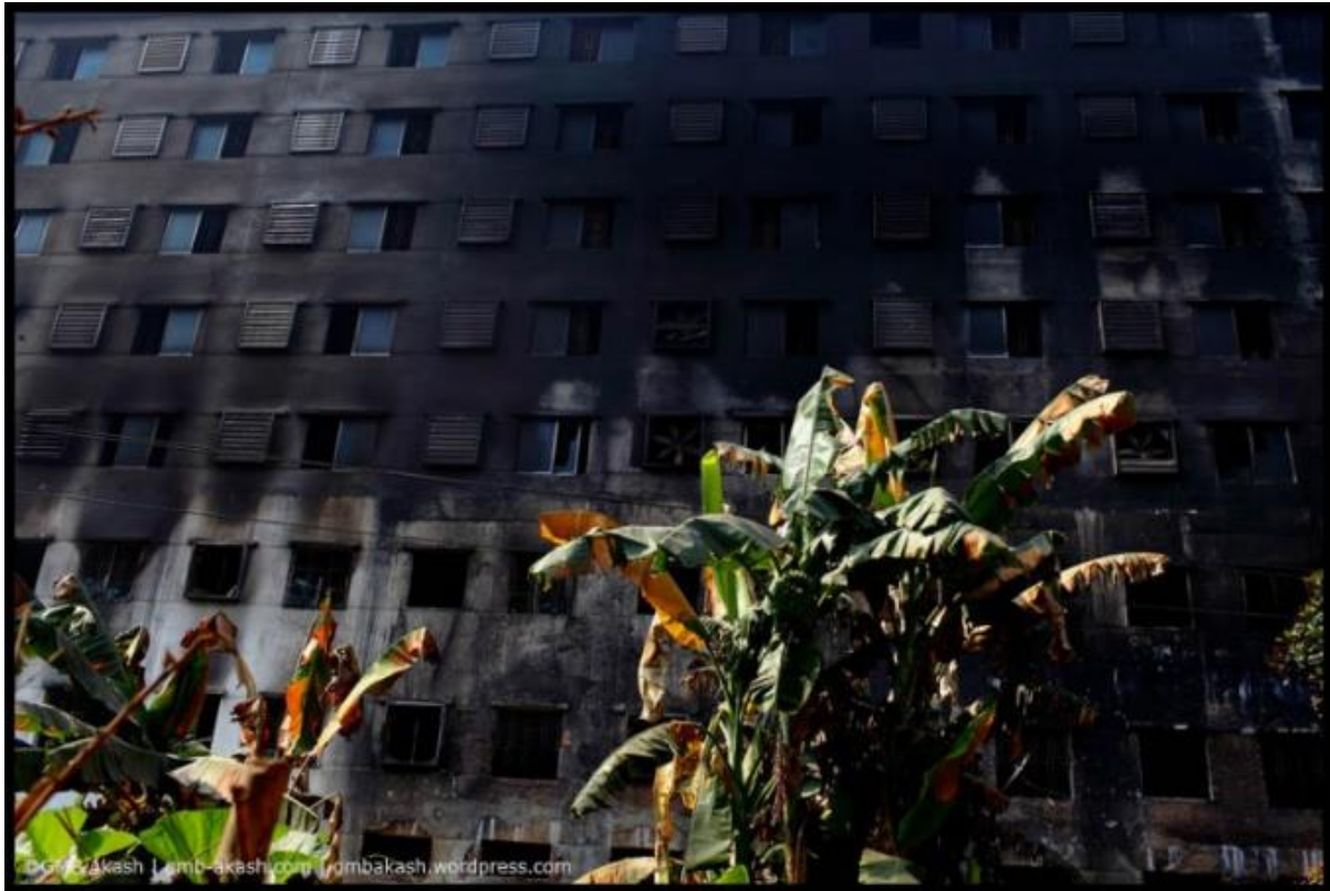
Figure 5: Tazreen Fashion Limited condition after fire hazard from outside (Akash, 2012).
