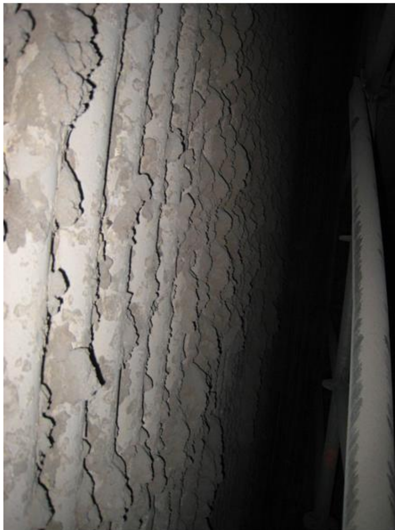
Figure 20. Slag formations on boiler wall tubes. (Andritz Oy's archives).
