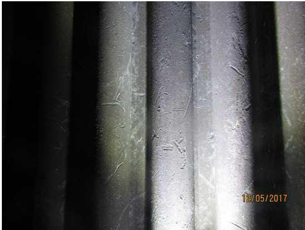
Figure 17. Ammonium corrosion. (Andritz Oy's archives)
