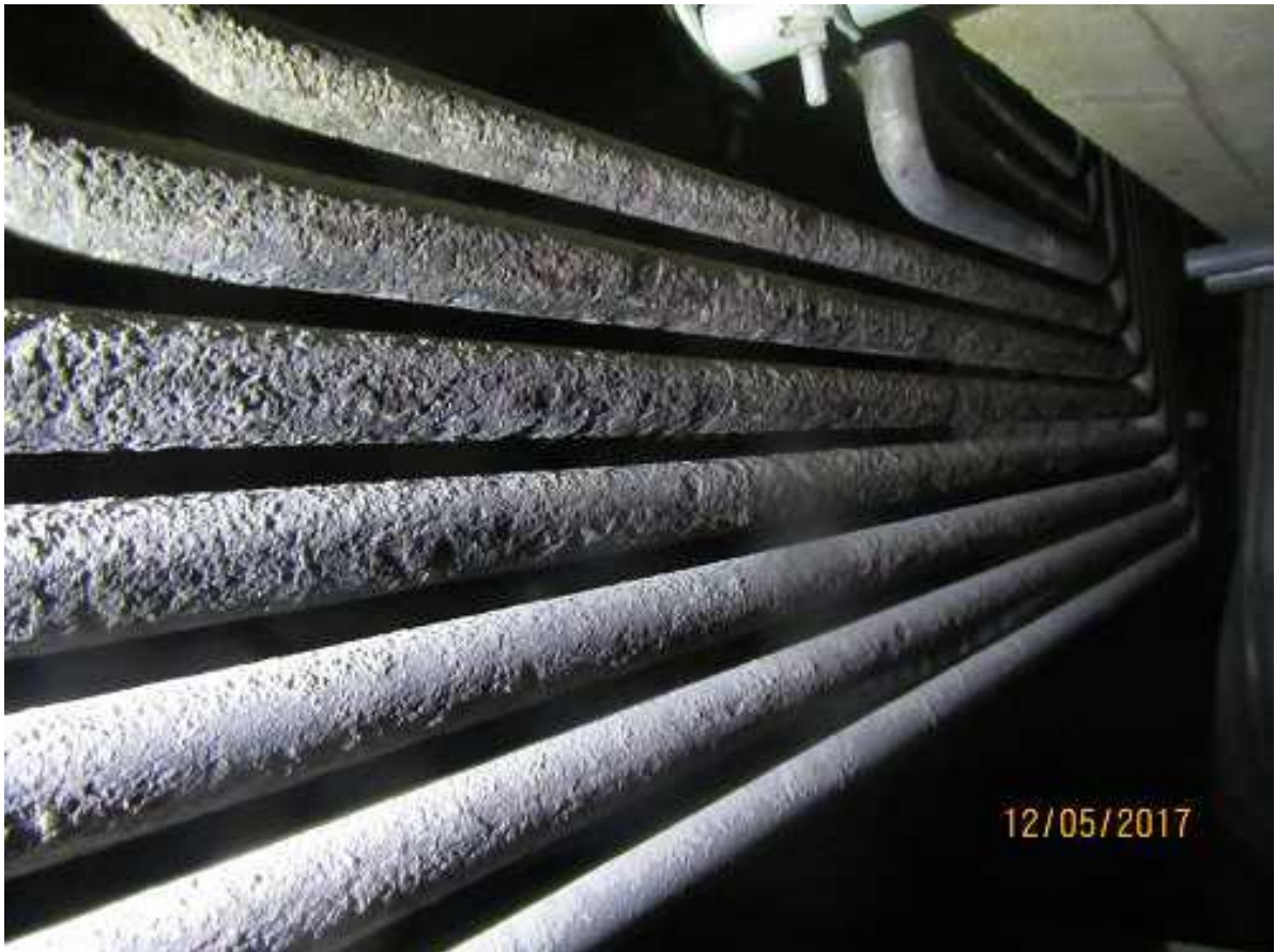
Figure 22. Hot corrosion on SH tube surfaces. (Andritz Oy's archives)
