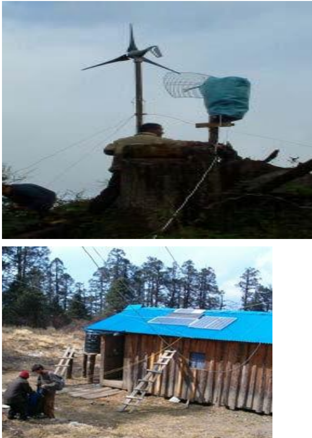
Picture 3. Wind Generator and Solar Panel [5].
