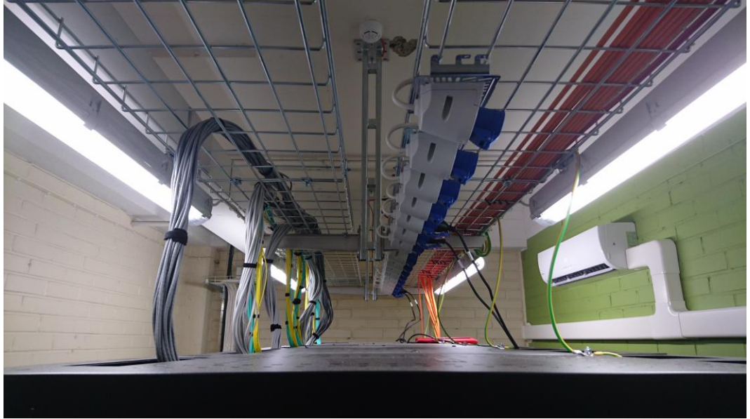
IMAGE 1. Rack overhead cabling
