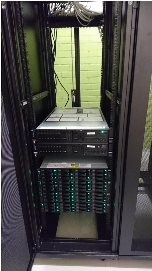
IMAGE 3. ESXi hosts and storage installed into a rack.
