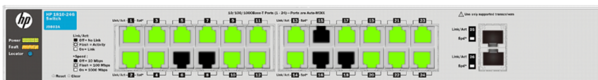
Image 2. HP 1810-24G switch ports in use.
