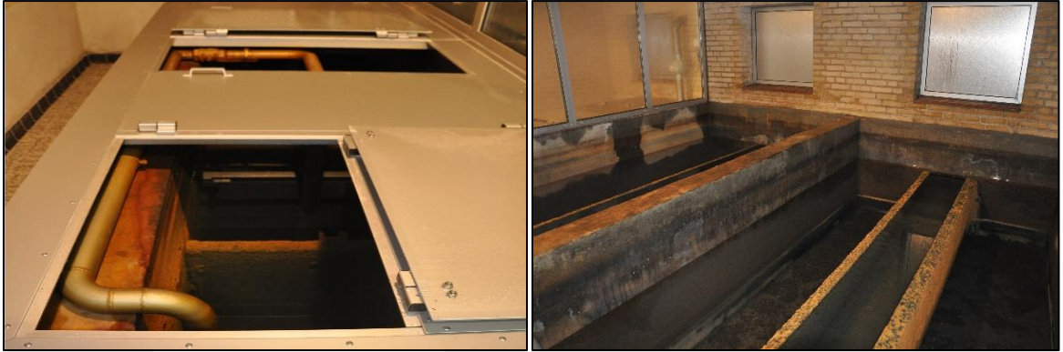
Figure 6. Aeration basin and sand filters in new waterwoks (Skovby waterworks 2016)
