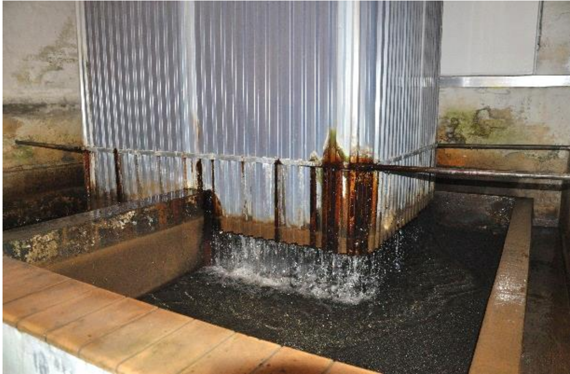
Figure 5. Free-fall aerator and sand filters in old waterworks (Skovby waterworks 2016)
