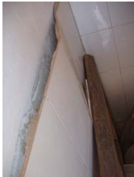
Figure 3-3 Bad Construction Quality
