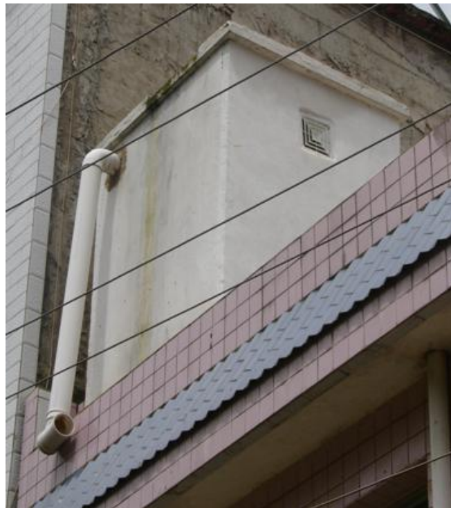
Figure 3-7 Poor construction quality or unprofessional construction (Photo by Ma Wenting)
