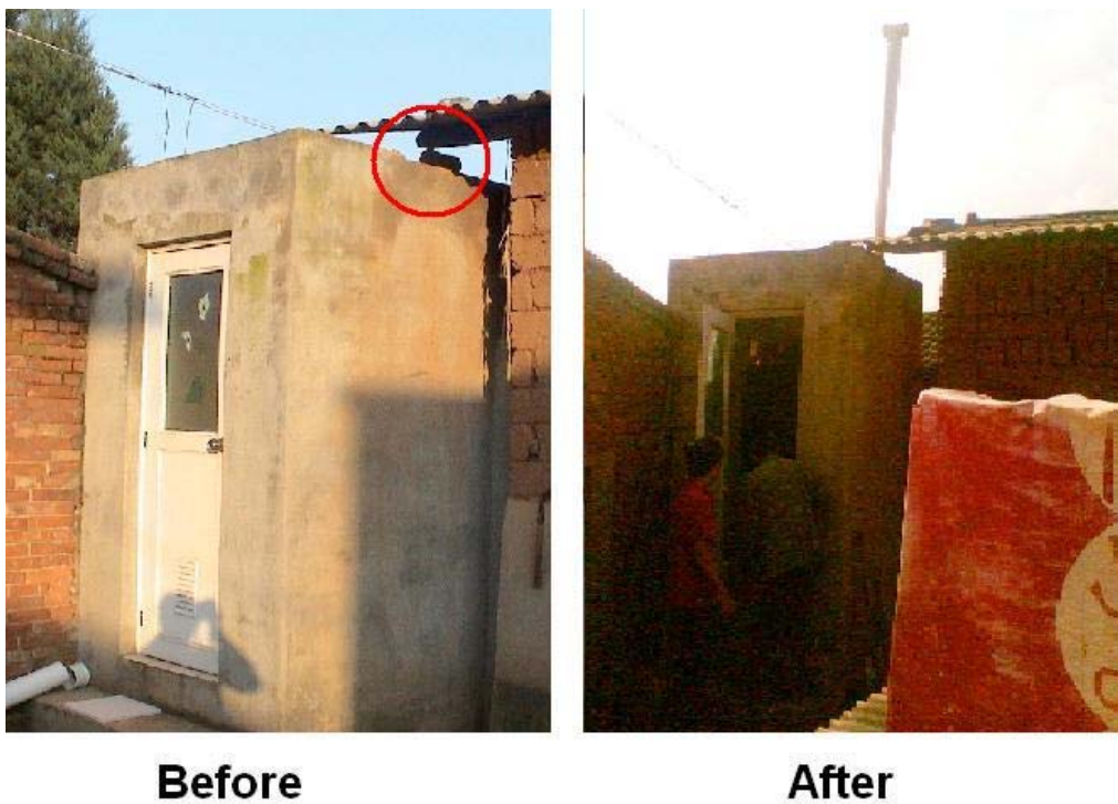
Figure 4-1 Ventilation Pipe Before and After Fixing
