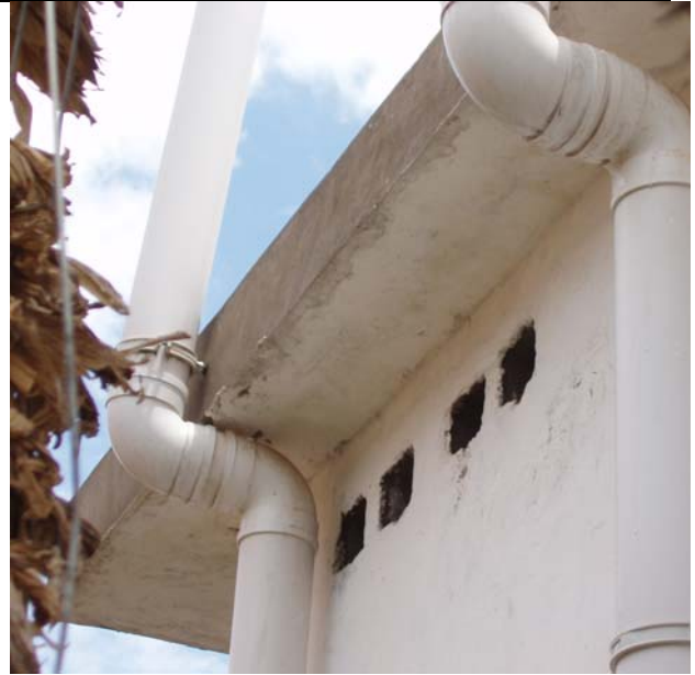
Figure 3-6 Ventilation pipe turning
