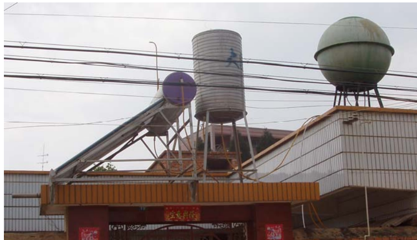
Figure 6- 4 The Solar Heating System
