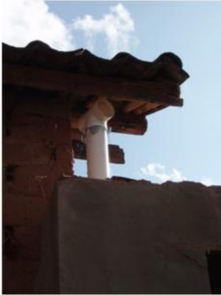
Figure 3-5 Short Ventilation pipe
