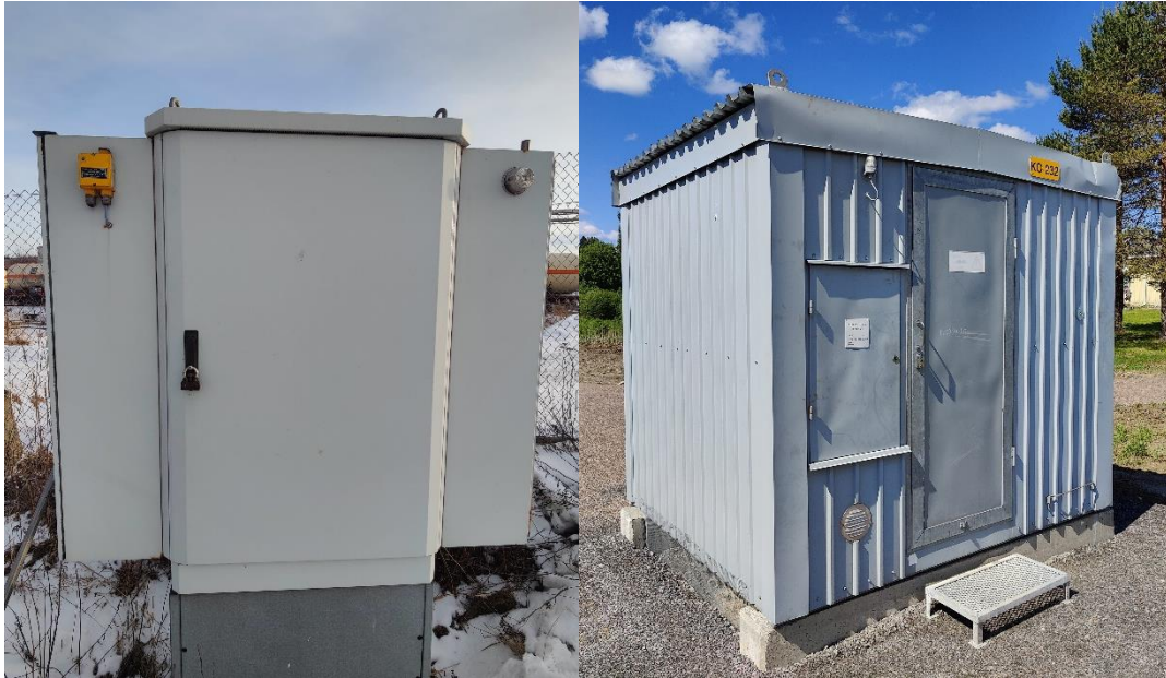
Figure 23. Track-Side equipment cabinet (Left) & equipment hut (Right)
