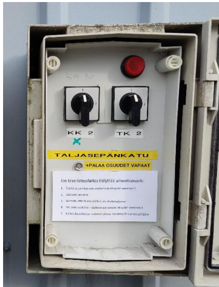
Figure 21. KK & TK Switches
