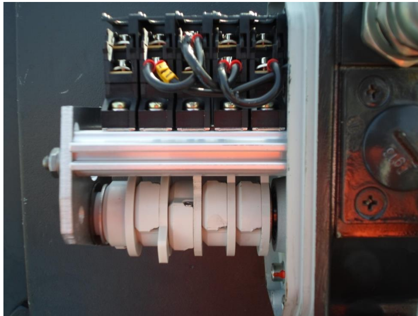
Figure 24 Hoist limit switch cams
