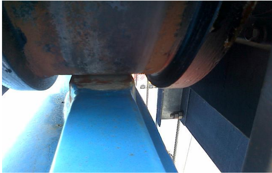
Figure 29 Trolley wheel on rail (still shows some gap on the rail)
