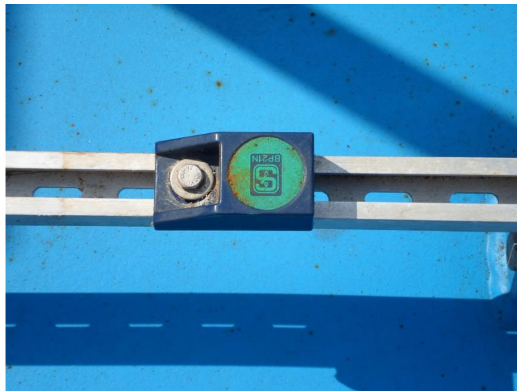
Figure 25 Trolley backward limit magnet
