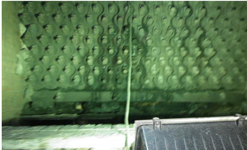
Figure 8. Water holes of the boiler at Samartex
