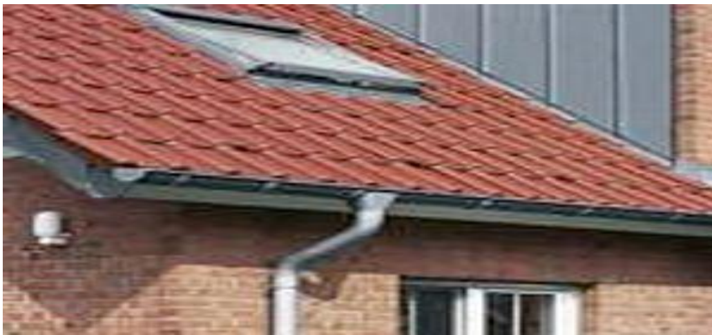
Figure 16: depicts a plastic roof and its drainage gutters
