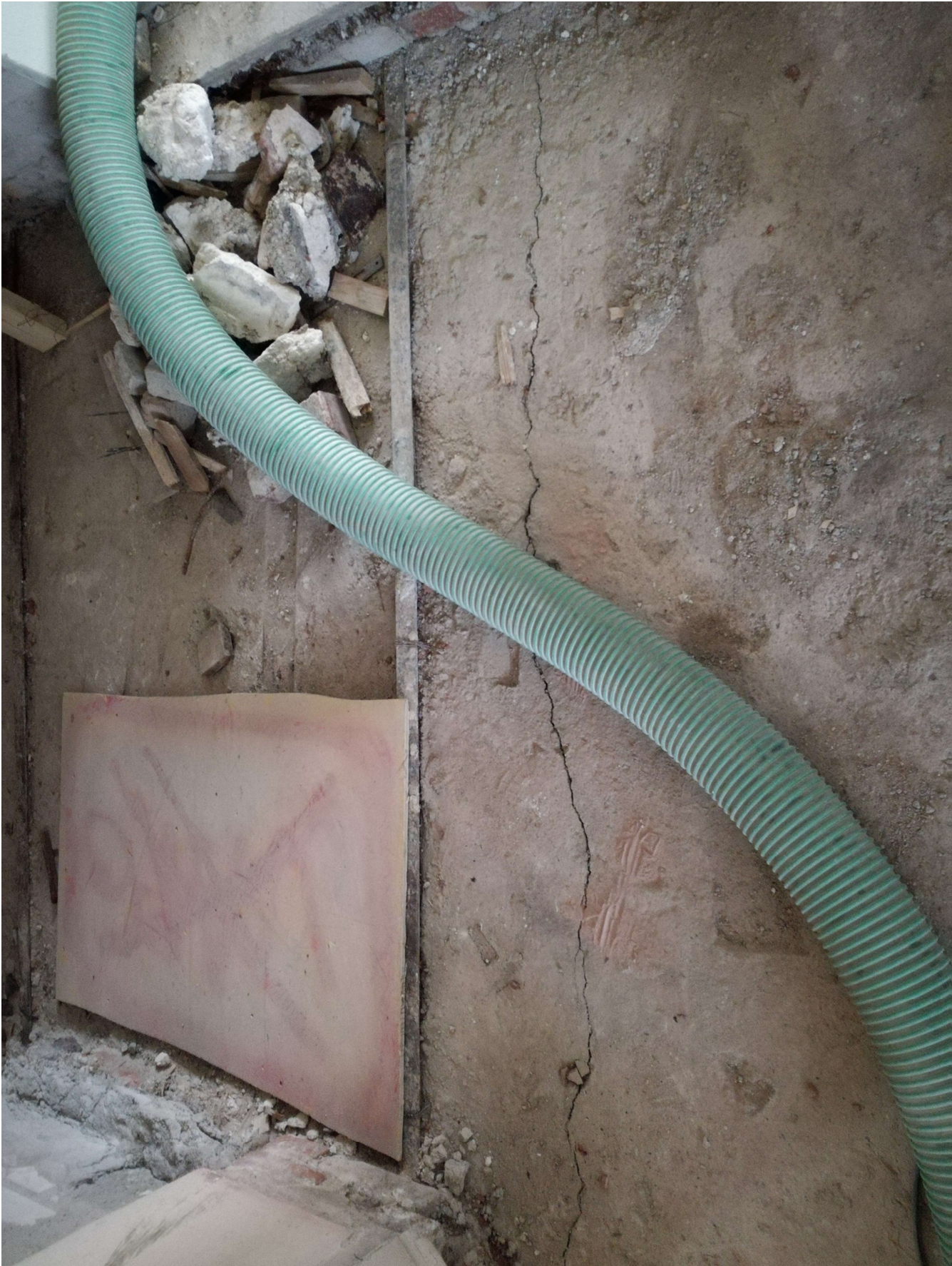
Appendix 1/1 Visible crack on the old concrete slab
