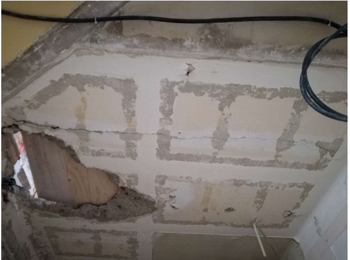
Figure 5. Cracked floor slab
