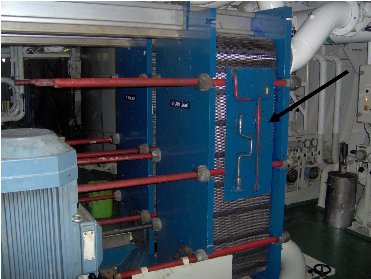
Picture from Estraden (Central cooler)
