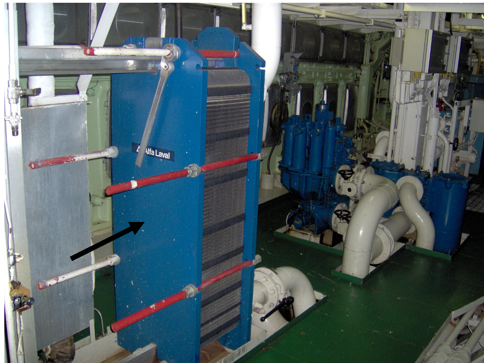
Picture from Estraden (Lubricating oil cooler)
