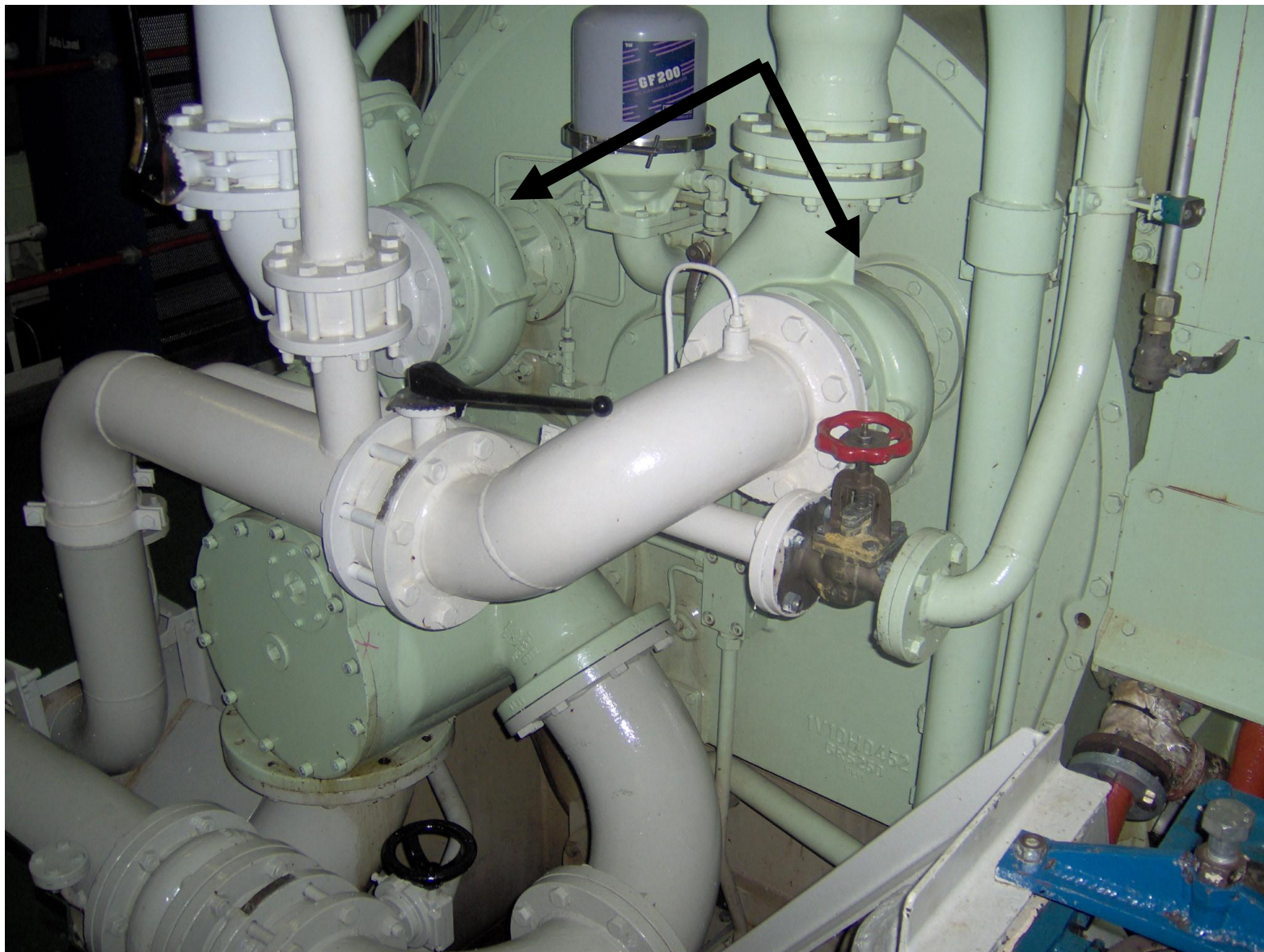
Picture from Estraden (Engine driven cooling pumps)
