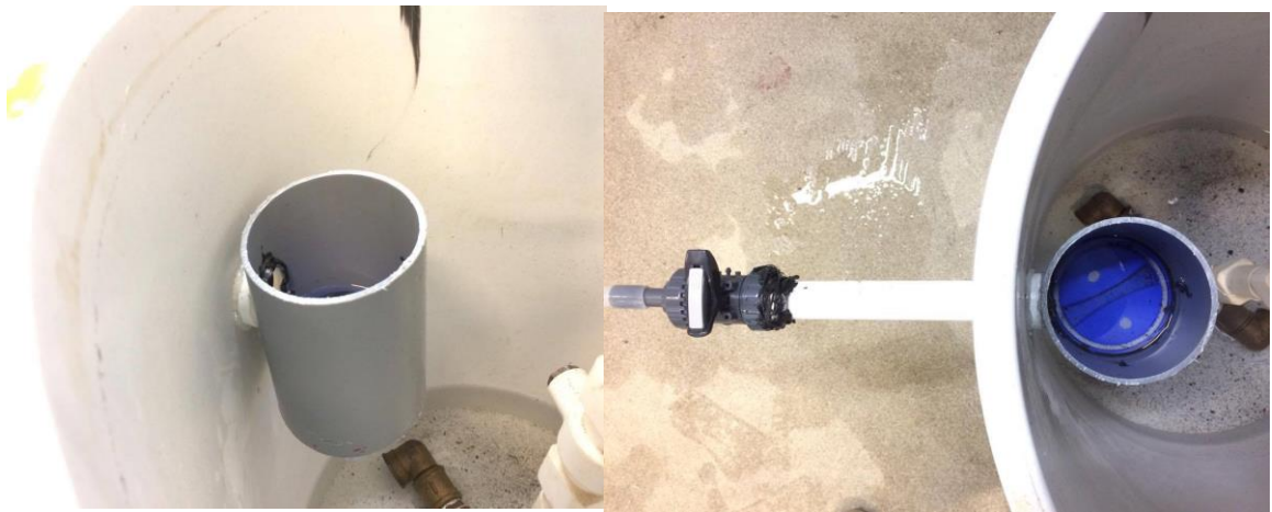
Figure 17. Weir and effluent design with section view (A) and plan view (B)
